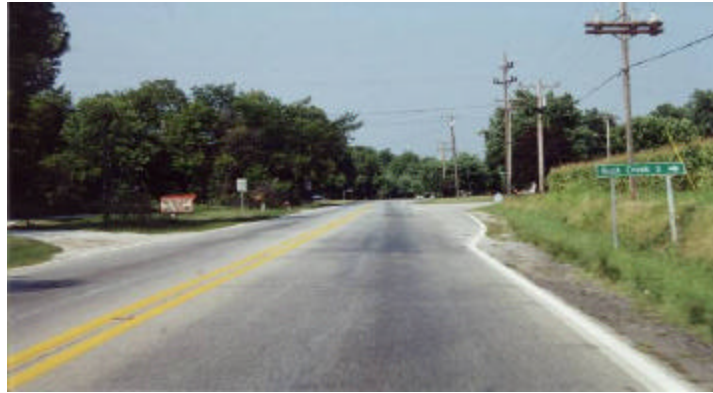
Figure 2: Lack of pavement markings or signing with auxiliary lanes
