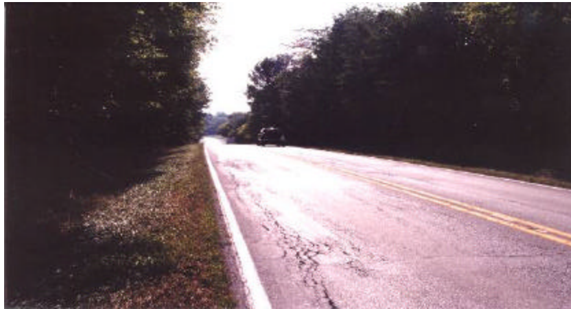
Figure 1: Lack of shoulder in the cross-section
