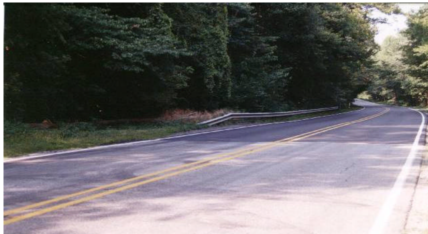
Figure 4: Example of one roadside barrier installation problem: Outdated terminal
