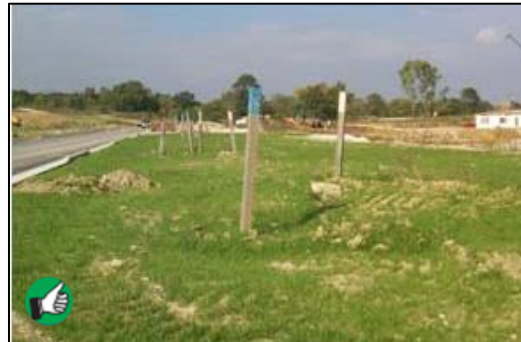
Example of temporary seeding to cover open areas where construction is not taking place.
