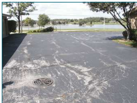
Parking lot showing worn and eroded sealcoat.
