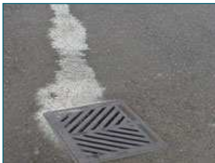
Erosion pathway from parking lot to storm drain
